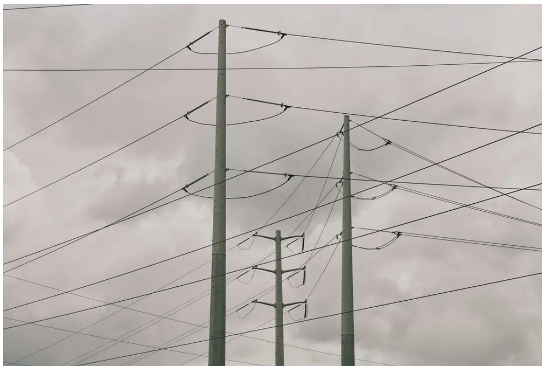
Power companies are spending more on new transmission lines, batteries, wind turbines, solar farms and other gear to reduce greenhouse gas emissions. Mason Trinca for The New York Times
